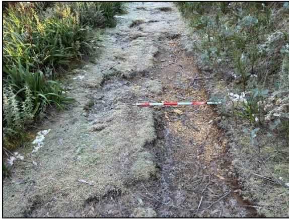
Plate 3. Eroded exposures along access track (northwest)
